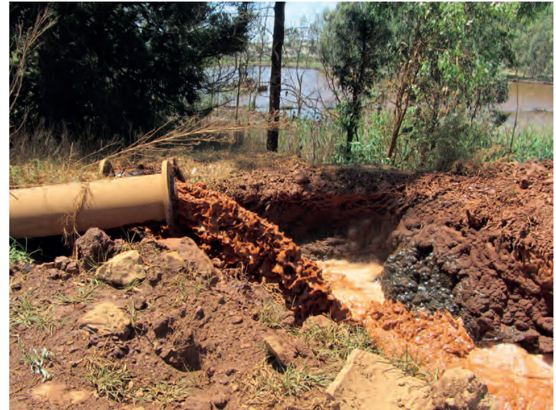
AMD neutralized at the West Rand Treatment Plant has flowed for several years through this pipe and manmade trench to a nearby pit, where heavy metals have precipitated. The water, which has continued on to the Tweelopiespruit in the background, however, has retained dangerously high sulfate levels. © 2014 Bonnie Docherty/IHRC.
