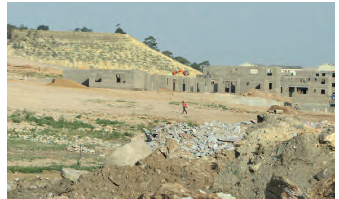
Homes were under construction at the foot of a tailings dam near Meadowlands in the Central Rand in 2014. The government should require a greater buffer between new residences and waste dumps. © 2014 Bonnie Docherty/IHRC.
