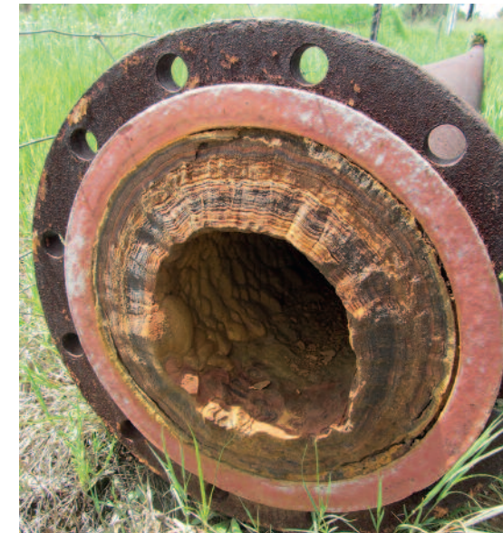
Layers of orange AMD residue have frequently accumulated inside steel pipes. These radioactive materials should be, but have not always been, deposited in a licensed storage facility. © 2012 Bonnie Docherty/IHRC.
