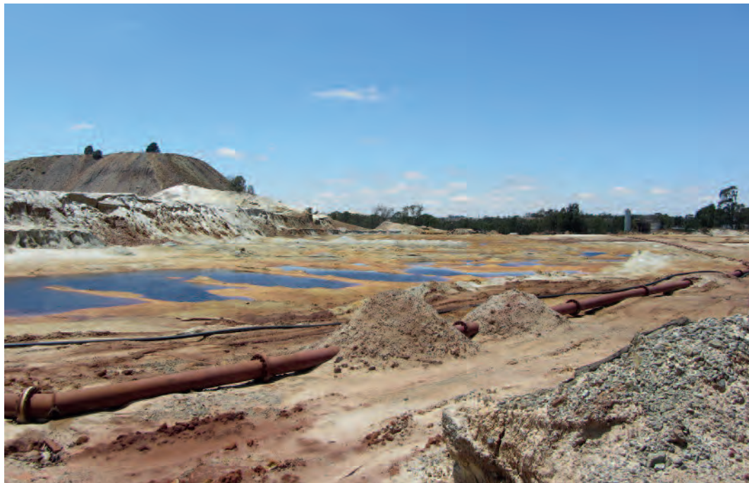
This remining operation, shown in 2014, had almost completely eliminated Sand Dump No. 20 by 2016. While such reclamation has helped address the tailings problem, it must be done carefully because the process stirs up contaminated dust. © 2014 Bonnie Docherty/IHRC.
